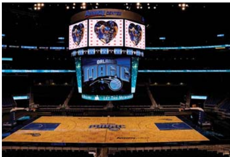
The digital signage at Amway Center, managed via a Harrisbuilt control room, presents a consistent look and feel to deepen the impact of brand messaging and announcements.
